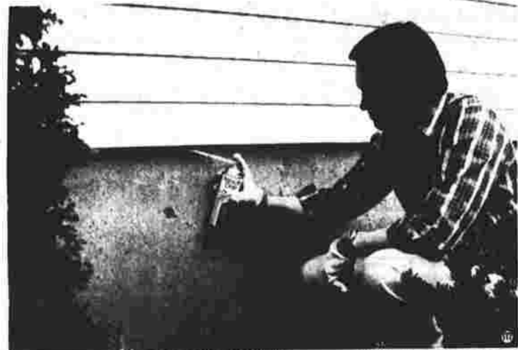
A HOMEOWNER APPLIES A FOAM SEALANT to an area which is the major culprit of energy loss, the soleplate where the frame and foundation of a house meet on an exterior wall.
